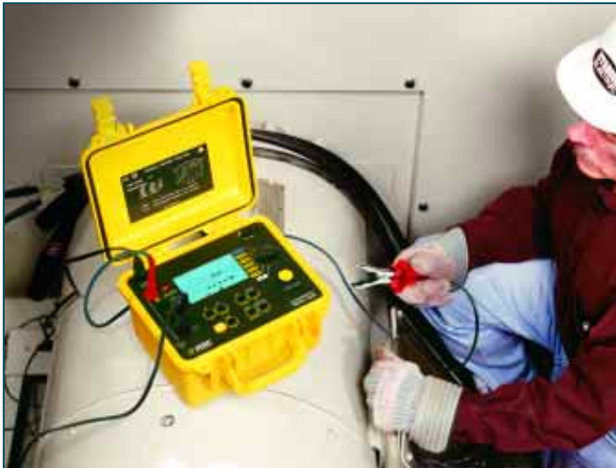
Model 5060 performing insulation test on a generator.
